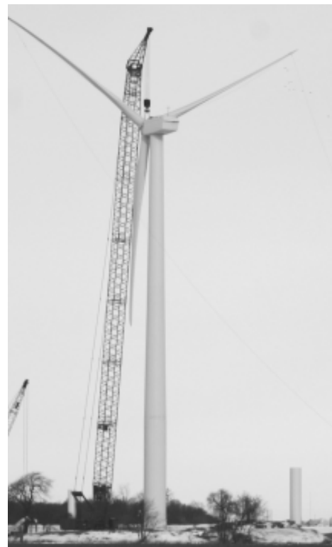
A crane lifts turbine components into place on a tower in the Blue Sky Green Field project in Fond du Lac County. The lower section of a tower rises in the background.
