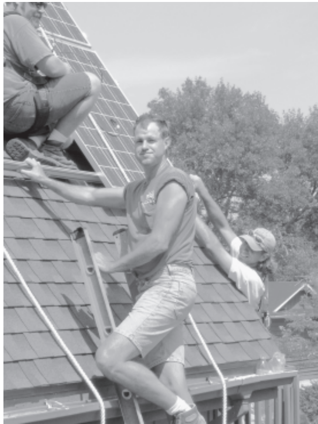
Andy Bangert works with Chad Silverthorn (on the roof) and Pete Bunch (behind Andy) on an installation at the home of Karl and Nina Loeffler just outside of Madison.
